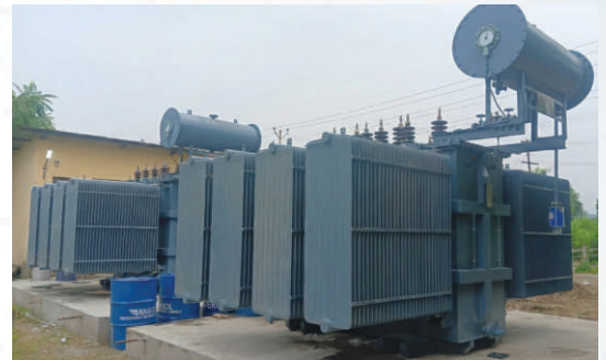
10 MVA PowerTransformer Installation (Actual Site Photo)
