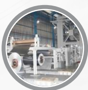
Aluminum Extrusion Plant
