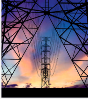
Transmission & Distribution Network
