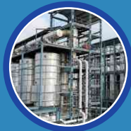
Distillery Power Plant
